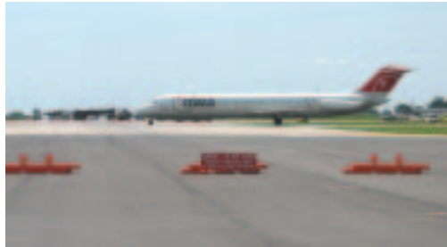
As a large Northwest Aircraft prepares for takeoff on an active runway, in the background you can see the entourage of construction vehicles working on the Runway Rehabilitation.
