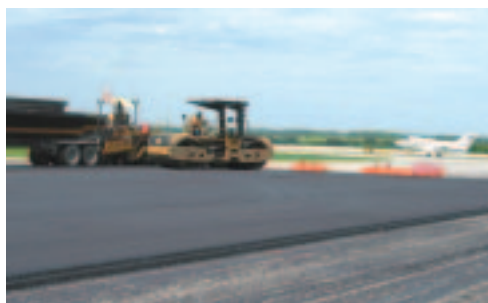
Two of the more than 200 workers utilized to complete the Runway 13-31 Rehabilitation Project are busy laying pavement right next to an active runway. Safety and extra care were paramount in finishing the project and not affecting the regular air operations on the crosswind Runway 5-23.
